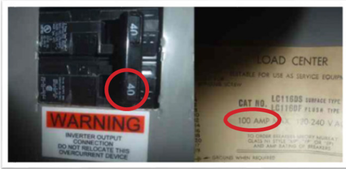
Photo 2: Backfed PV breaker not installed at opposite end of buss bar from main breaker: NEC 705.12(B)(3)(b)
