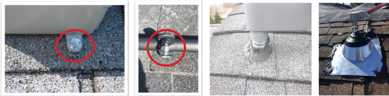
Photo 7: Where not protected from physical damage, equipment grounding conductor must be #6 or larger: NEC 690.46, 250.120(C). Conductors laying on asphalt shingles will become damaged and will not last a PV system's expected 30-year lifespan.
