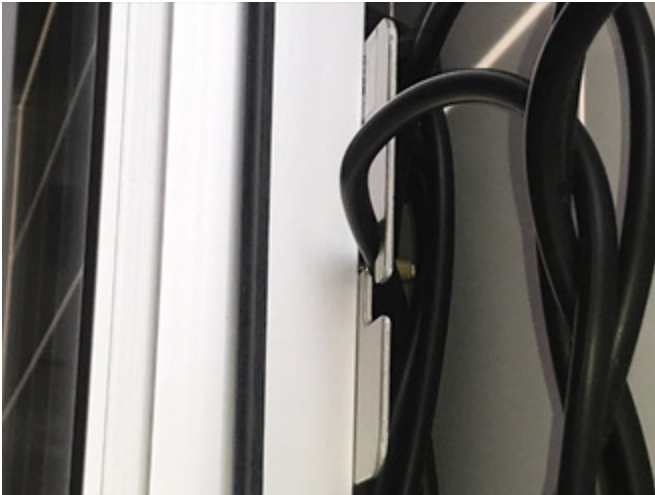
Photo 10: DC Conductor in contact with sharp edge: NEC 334.15(B)
